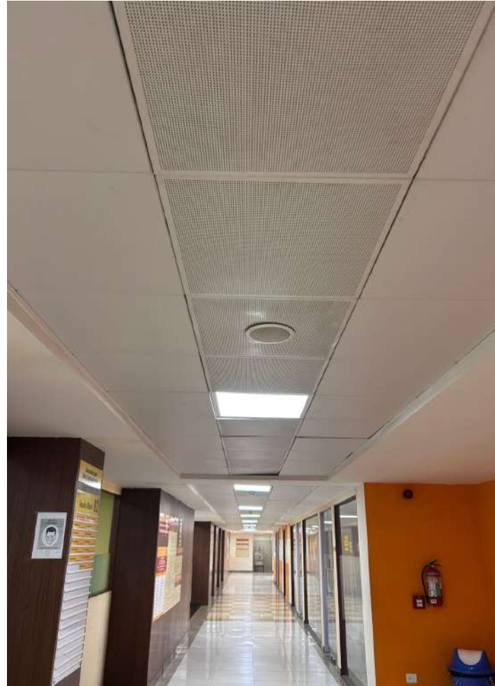
Efficient Heating and Cooling
